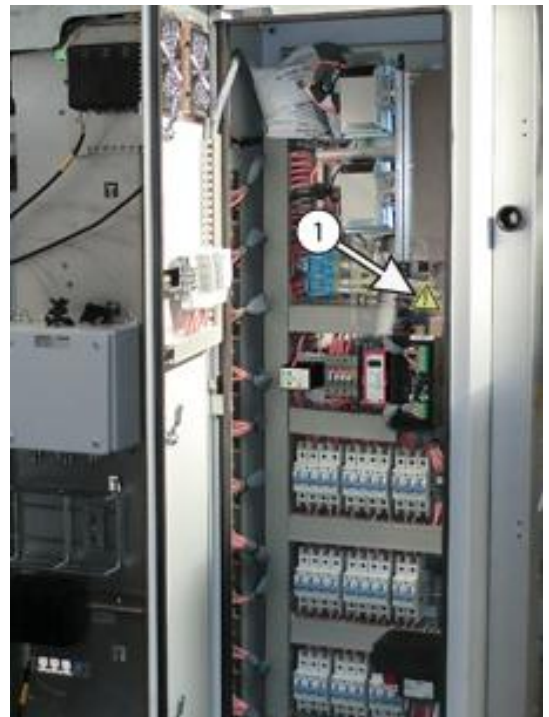
Figure 16-6: Inside of the auxiliary power supply on plexiglass
