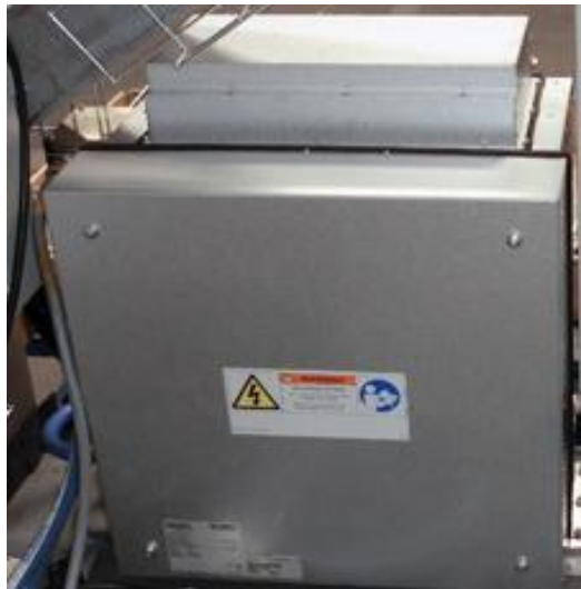
Figure 16-10: 119442 - Hazardous voltage - LOTO procedures required on the control module
