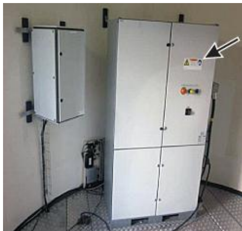
Figure 16-2: 119442 - Hazardous voltage - LOTO procedures required on the tower control cabinet
