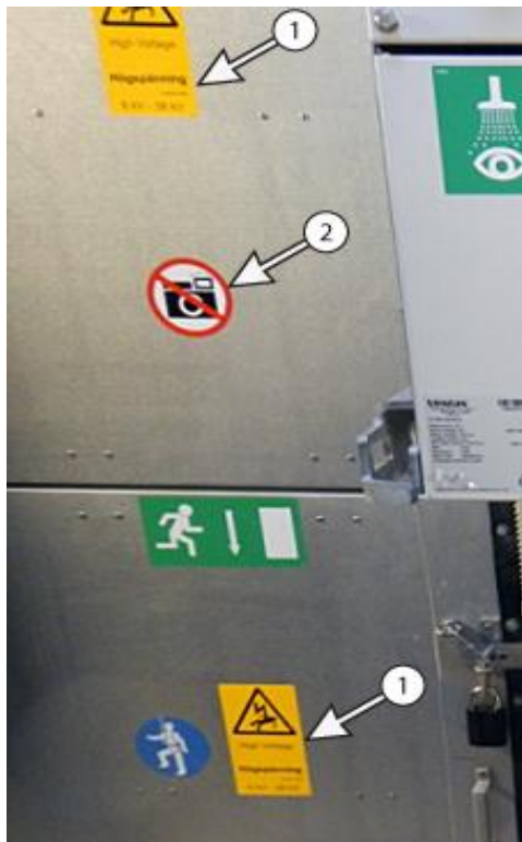
Figure 16-7: Additional transformer door signs
