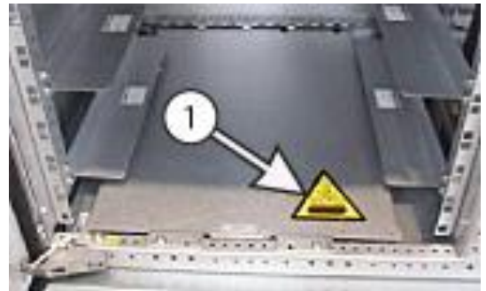
Figure 16-4: Under UPS location in the tower control cabinet
