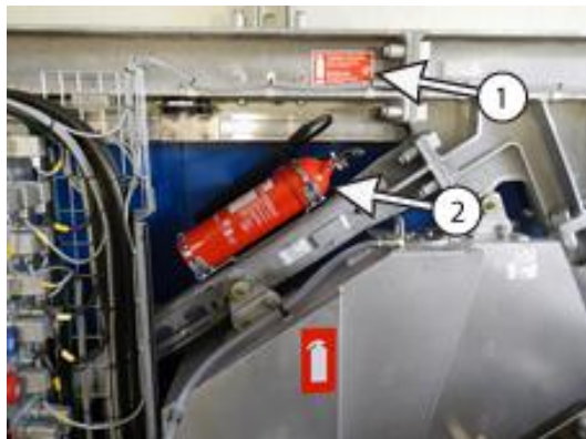
Figure 16-20: Fire extinguisher location
