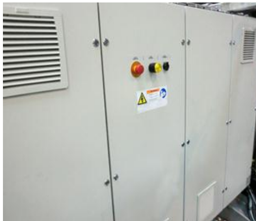
Figure 16-11: 119442 - Hazardous voltage - LOTO procedures required on the nacelle control cabinet
