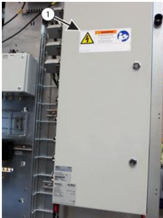
Figure 16-5: Outside on the auxiliary power supply
