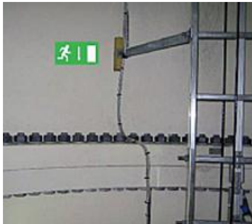
Figure 13-4: 208015 - Emergency exit (arrow down)
