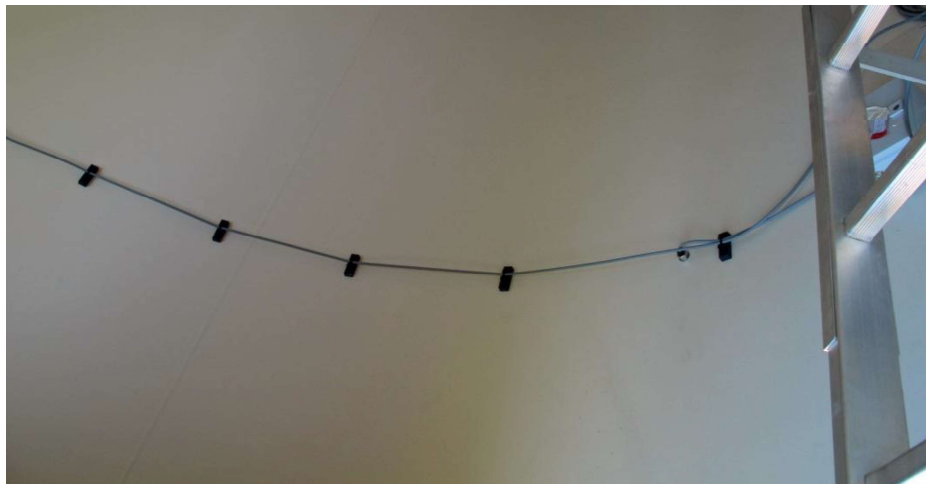
Figure 3-2: Cable routing inside the tower
